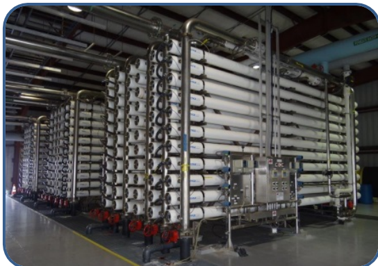
Reverse Osmosis Trains
